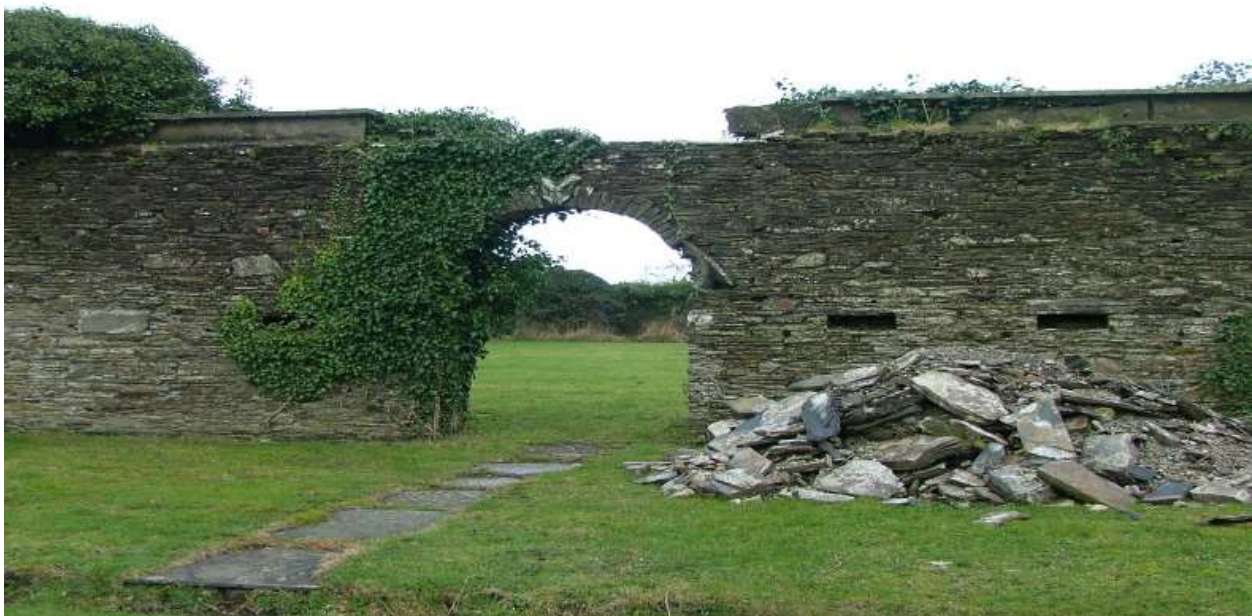
Walled garden at Tredethy House near Bodmin, some demolition has already taken place.
